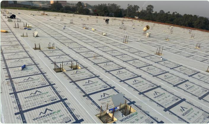
Cold Storage and Cold Room
